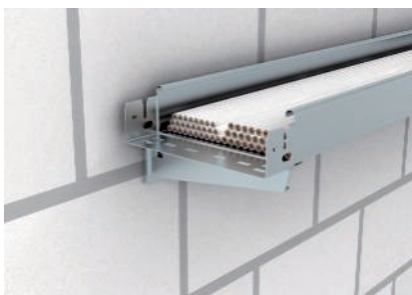
Reference laying type: C Cable on unperforated cable tray, e.g. type MKSMU
